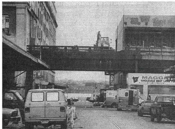
A demolition crew at Gansevoort St. where the High Line was finally truncated
